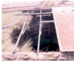
h01889 gisborne mains house cistern
