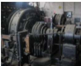
Substation - Rotary converters
