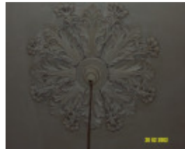
23435 Skene Homestead Strathkellar 1858 hall ceiling 1585
