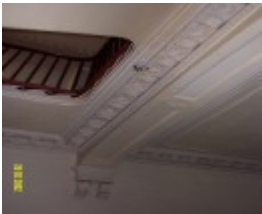
23435 Skene Homestead Strathkellar 1858 hall ceiling 1583
