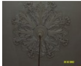
23435 Skene Homestead Strathkellar 1858 hall ceiling 1585
