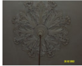
23435 Skene Homestead Strathkellar 1858 hall ceiling 1585
