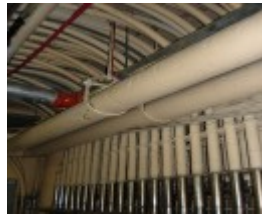
Myers Melbourne Lamson Tubes Ceiling February 2006
