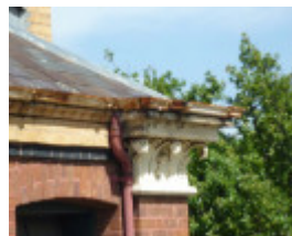
Before Photograph - Reference F3838 2014
