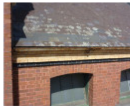
Before Photograph - Reference F3838 2014
