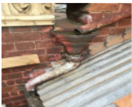
Before Photograph - Reference F3838 2014
