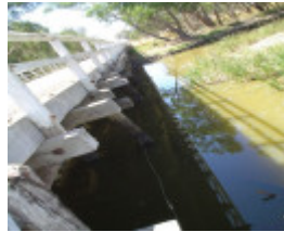
h01850 danns bridge over bet bet creek dunolly eddington road eddington railings she project 2004
