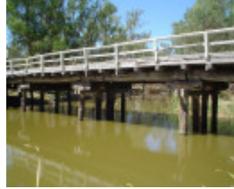
h01850 1 danns bridge over bet bet creek dunolly eddington road eddington close view she project 2004
