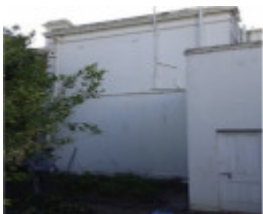
Before Photograph - Reference F3856 2014
