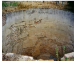
MAW 01 2 - Photograph, Brick lined underground tank - Shire of Northern Grampians - Stage 2 Heritage Study, 2004
