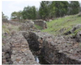
Partial collapse of Bessiebelle July 2013
