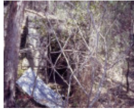
h01556 heatherlie quarry grampians national park halls gapp stone powder magazine she project 2004
