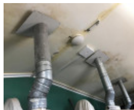
Memorial Hall Koroit, projector chimneys.JPG
