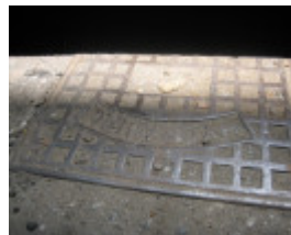
H2117 Overhead Water Tank Spencer St Power Station Hydraulic Valve Cover Plate 6 Dec 2006 mz
