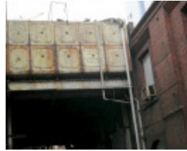
OVERHEAD WATER TANK SOHE 2008
