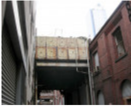
OVERHEAD WATER TANK SOHE 2008
