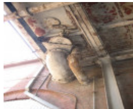
H2117 Overhead Water Tank Spencer St Power Station Outlet Pipe and Valve 6 Dec 2006 mz
