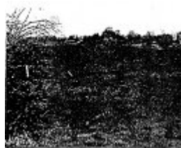
Railway Conservation Precinct - View of railway line embankment and brick culvert - 1983 Buninyong Conservation Study
