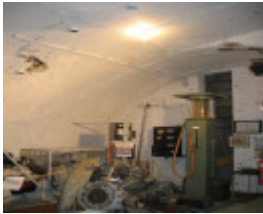
Internal view of engine room, Feb 2008.
