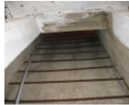
Looking up the escape hatch and air shaft at western end of building, Feb 2008.
