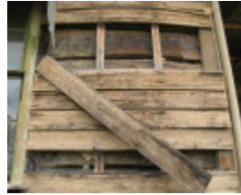
Castlemaine military quarters_slabs under weatherboards_KJ_7 Feb 08
