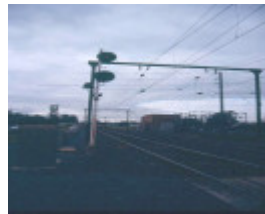
h02025 7 bunyip sub stationjul03 jc
