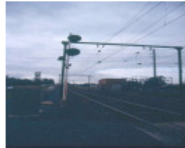
h02025 7 bunyip sub stationjul03 jc
