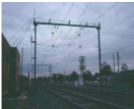
h02025 6 bunyip sub stationjul03 jc
