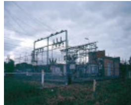
h02025 4 bunyip sub stationjul03 jc1
