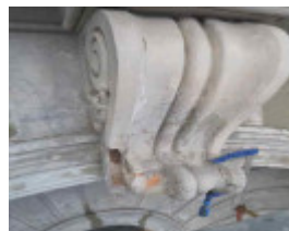
Before Photograph - Reference F3924 2014
