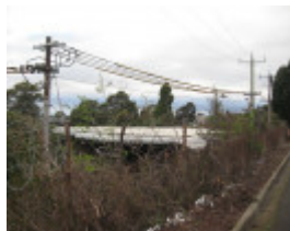
Maribyrnong substation view from above
