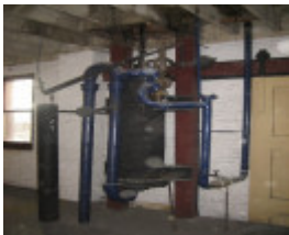
61-9 A'Beckett St lift ground floor MZ 24 05 2007
