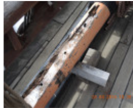
Before Photograph - Reference F3930 2014
