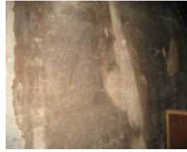
2010_Oct_1_Black Eagle_wallpaper remnants
