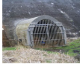
The western valve house.jpg
