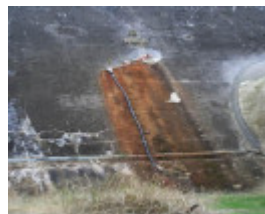
Crack in the dam wall.jpg
