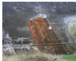
Crack in the dam wall.jpg
