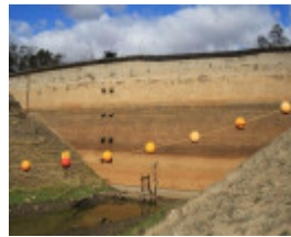
The inner face of the Lower Stony Creek Dam Wall showing some water in the reservoir.jpg
