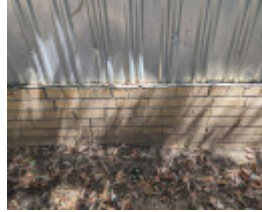
Damage to building
