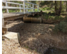
Build-up of material in waterway/under bridge
