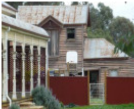
East elevation of the stables, with the verandah of the presbytery at right.
