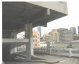
Total House office supports
