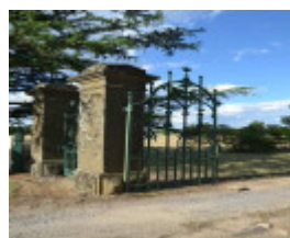
Photo 5 Pillar showing slight damage and rotation.jpg
