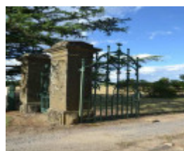
Photo 5 Pillar showing slight damage and rotation.jpg
