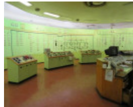
View inside the Power Station Control Room.
