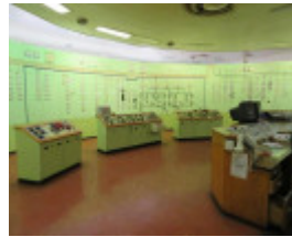
View inside the Power Station Control Room.
