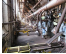
View of conveyors leading from briquette machines to external conveyor, looking east.
