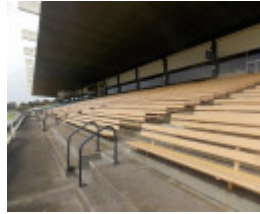
Detail of seating area, showing stepped concrete tier, bench seats and canopy underside.jpg
