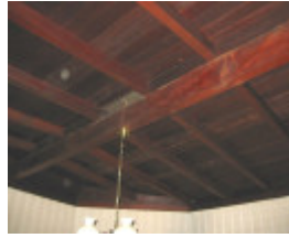
h01009 desbrowe annear house 38 the eyrie eaglemont lining room ceiling air vent feb mz
