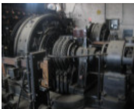
Substation - Rotary converters
