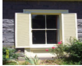
23187 Warrayure Homestead Complex window 1884
