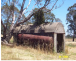
23254 Timber Kiln and Boiler Balmoral 2095
