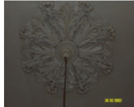
23435 Skene Homestead Strathkellar 1858 hall ceiling 1585
