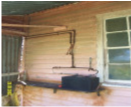
23526 Hillview Nareen electrical system 1982
