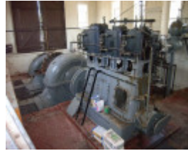
LOCK NINE PUMPING STATION SOHE 2008
