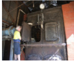
LOCK NINE PUMPING STATION SOHE 2008
