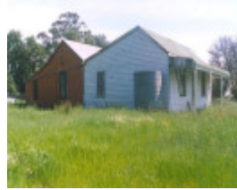
205904_Derrinal_Sheedys Lane_Murrowood Homestead_img02 photo prior to fire. The timber part is now destroyed as is the roof structure of the brick part.
