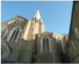
Before Photograph - Reference F3890 2014
