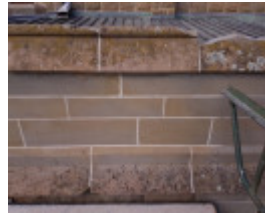
Before Photograph - Reference F3890 2014
