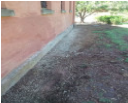
Before Photograph - Reference F3878 2014
