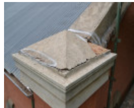
Before Photograph - Reference F3878 2014
