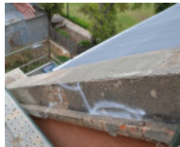
Before Photograph - Reference F3878 2014
