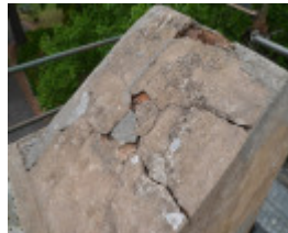
Before Photograph - Reference F3878 2014
