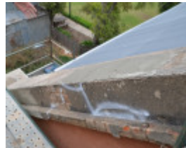
Before Photograph - Reference F3878 2014
