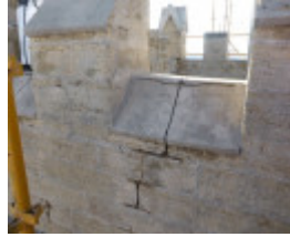
Before Photograph - Reference F3866 2014
