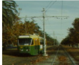
1 ornamental tramway overhead poles dandenong road
