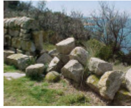
h01983 pt hicks drywall damage1 sep03 pm1
