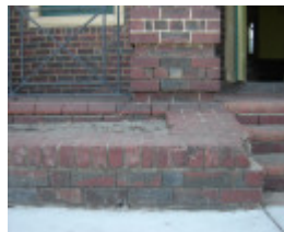
H1343 Exterior - East (front) facade, dislodged brickwork and missing mortar. Dec 2006.
