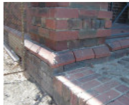
H1343 Existing condition - Exterior, south-east corner, dislodged brickwork and missing mortar. Dec 2006.
