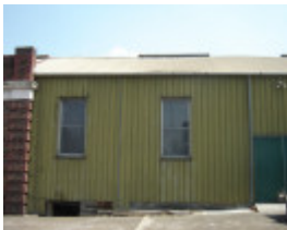
H1343 Exterior - North facade, note sagging roof sheeting. Dec 2006.
