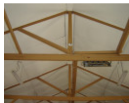
H1343 Interior - roof truss at east end of hall with missing strut. Dec 2006.
