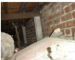
H1343 Subfloor, at shed hall to brick front junction. Dec 2006.
