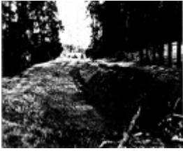
2 - Maroondah Aqueduct Kangaroo Ground Eltham N15 - of Eltham Heritage Study 1992 - Section of Aqueduct at Research that has been removed/filled in and replaced by a pipeline. A tunnel began/begins here. The surviving radiata pine tree plantings
