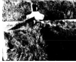
2 - Maroondah Aqueduct Kangaroo Ground Eltham N07 - Shire of Eltham Heritage Study 1992 - Silver pipe carries groundwater from abutting land over the aqueduct
