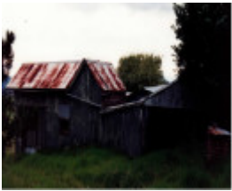
Garden Hill Shearing Shed Elth Yarra Glen Rd Colour 2 - Shire of Eltham Heritage Study 1992
