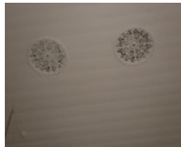
State school 2828 ventilators in ceiling KJ 26 Jul 07
