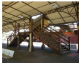
Access stairs to footbridge viewed from the southwest - from beneath the Platform 2 and 3 canopy
