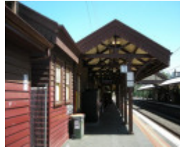
Looking southward along Platform 1 at its buildings and canopy - the canopy timber king-post trusses and support brackets of bent rail are visible
