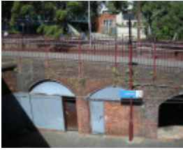
The northern-most of the arched alcoves beneath the pedestrian walkway have been enclosed to create storage areas
