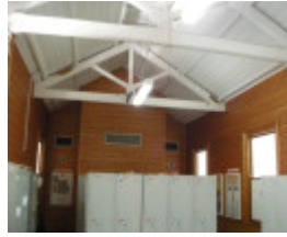
Looking north-east within the Burwood Rd end of the Platform 1 building - the king-post roof trusses about those of the platform canopy outside the wall to the left
