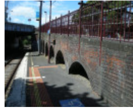
Looking north along Platform 3 at the west-facing brick wall beneath the walkway
