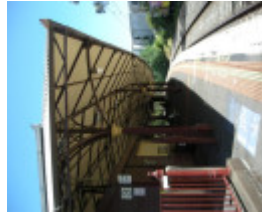
Looking from the north along the edge of Platform 3 - the matching curvature of the canopy roof and platform edge is evident
