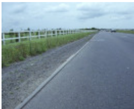
1 market gardeners tram plateway centre dandenong road heatherton front view of road
