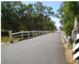
h01850 danns bridge over bet bet creek dunolly eddington road eddington across bridge she project 2004
