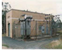
Wattle Glen railway 50hz electricity substation Colour 1
