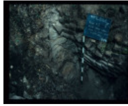
BATS RIDGE FAUNAL RESERVE, LIME KILNS FEATURE - KILN # 3 INSIDE VIEW, WALL DETAIL OF VENT HOLE AND LEFT WALL
